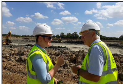
Northstowe – £49m infrastructure contract delivering, 400 units marketing progress, MMC office in construction
